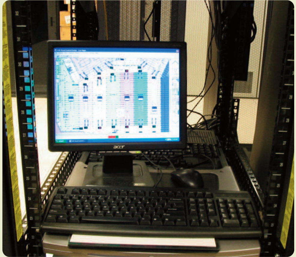
PGS server with level overview GUI in server room.
