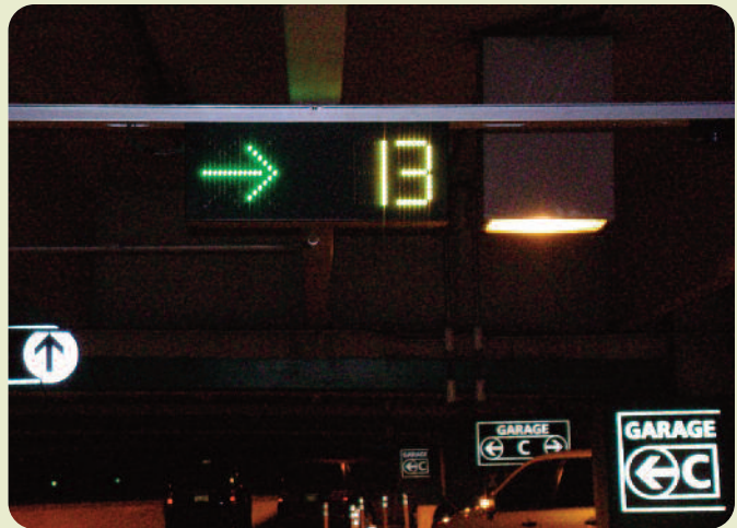
End of aisle directional signs display open spaces down each drive aisle.
