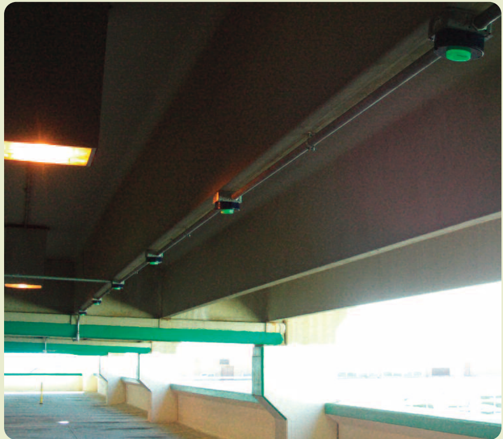
Single space sensors installed at perimeter and handicapped parking spaces.
